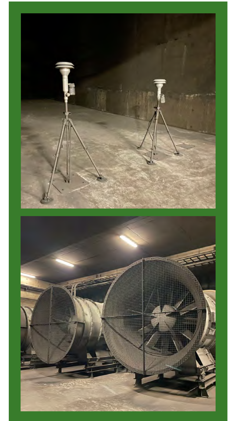
Pictured below: particulate matter sensors inside the stack (top); exhaust fans to extract tunnel air through the stack (bottom)
